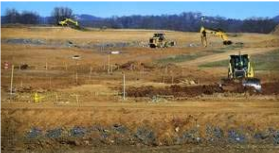
Purchase Image Zoom Construction equipment makes room for the Berry Farms subdivision in Franklin. Williamson County has seen the biggest percentage increase in housing starts. / Jae S. Lee / The Tennessean
